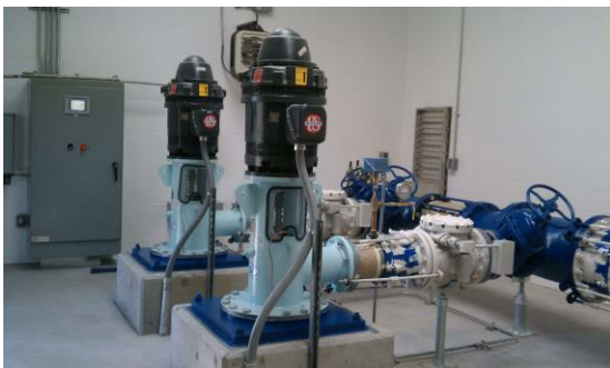
Prairie Ridge Booster Pumps
