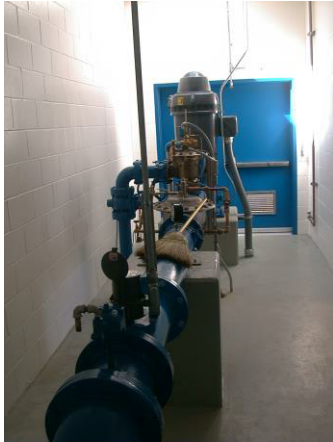
Tacoma Point Well No. 6
