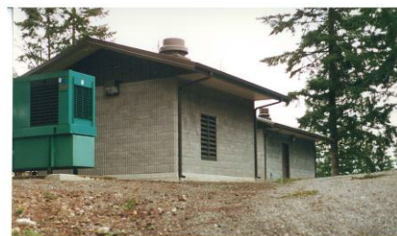
Ponderosa Booster Pump Station
