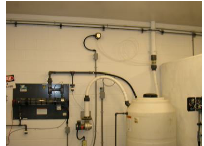
Grainger Springs On-site Chlorine Generator
