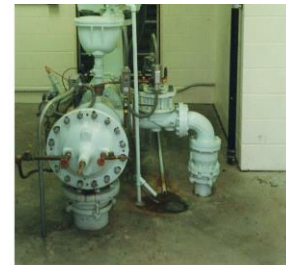
Tacoma Point Well No.4
