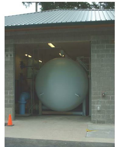
Ball Park Pressure Tank
