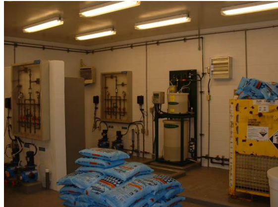
Grainger Springs Treatment Facility
