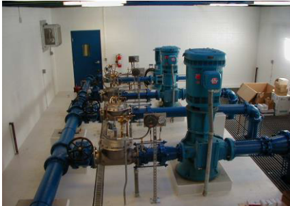
Lakeridge Booster Pumps
