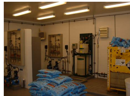
Grainger Springs Treatment Facility
