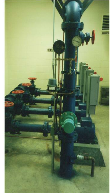
Ponderosa Booster Pump Station
