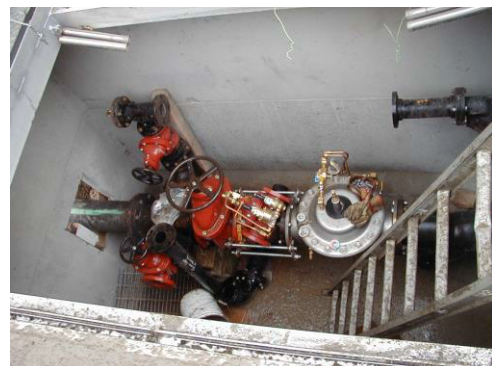
Cedar View Pressure Relief Station
