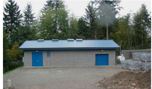
Lakeridge Booster Pump Station
