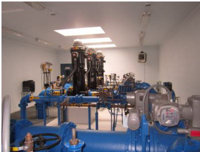
Peaking Storage Booster Pumps
