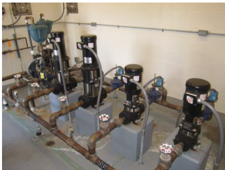
Panorama Heights Booster Pumps
